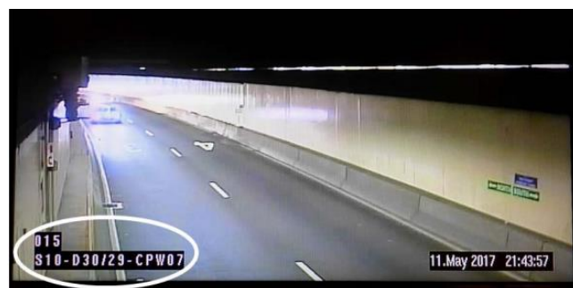
SOUTHBOUND TUNNEL DELUGE ZONES 30/29 CROSS PASSAGE 7
